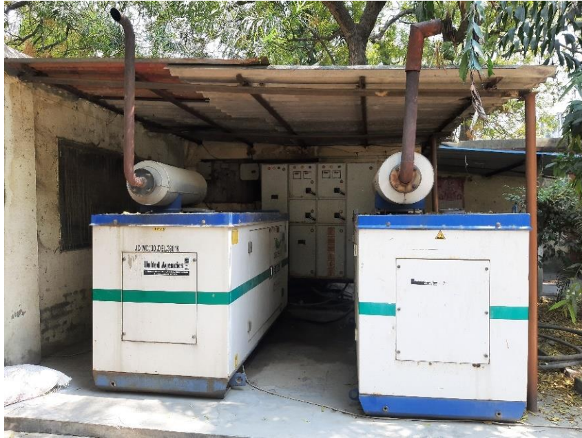
Figure 4: DG sets for electricity backup
