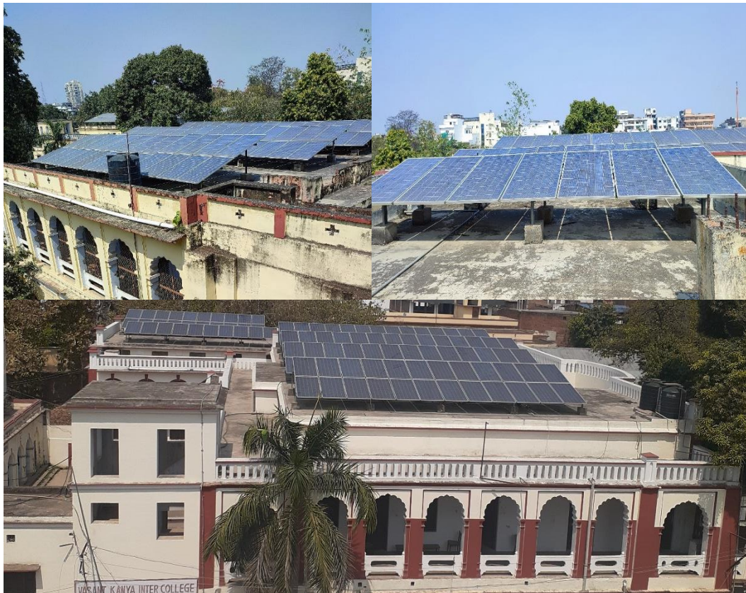
Figure 5: Rooftop Solar Panels
