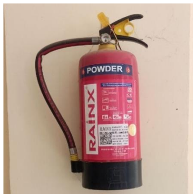
Figure 7: ABC-MAP 90 type Fire Extinguisher installed at each floor of the campus building
