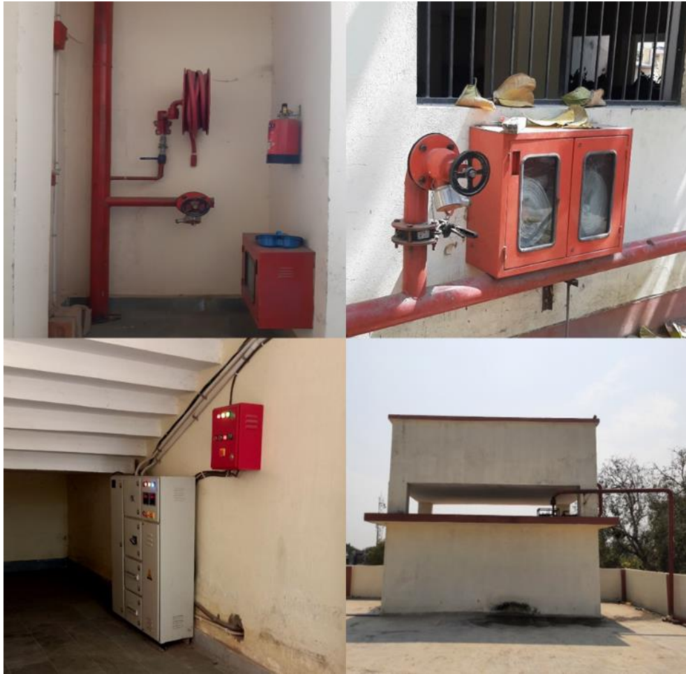
Figure 8: Fire Fighting System installed in Leela Sharma Block of VKM
