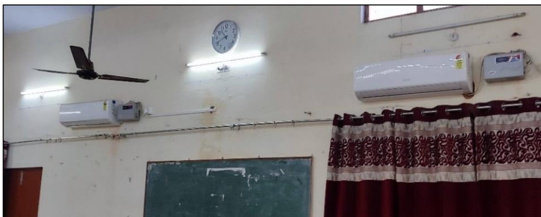
Figure 6: Energy saving 3-star AC installed in the Hall
